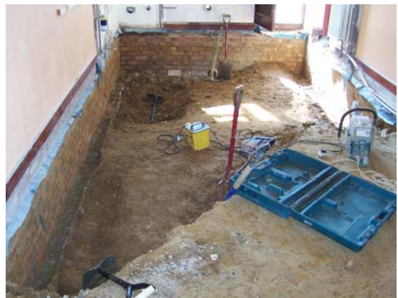
Kitchen floor and soil below removed because of oil contamination.
